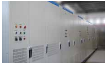
• Inverter to accompany in test
