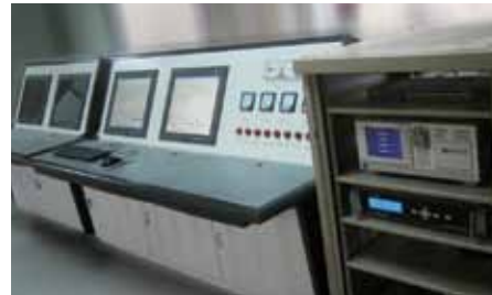
• Central control room
